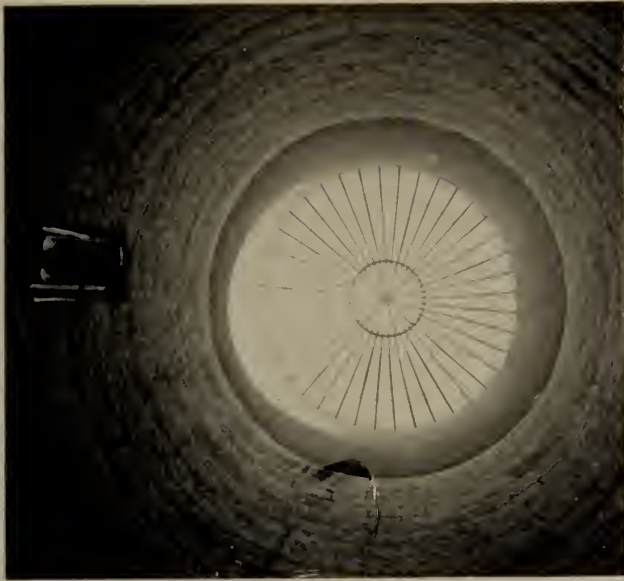
THREE GUESSES Photographer had holiday inside new "million dollar" waste burner at Shevlin-Hixon mill, Bend, Oregon. Camera points up toward steel screens. Ventilators like the one shown were built into firebrick 4 feet thick. (Photo by Ray Van Vleet)
